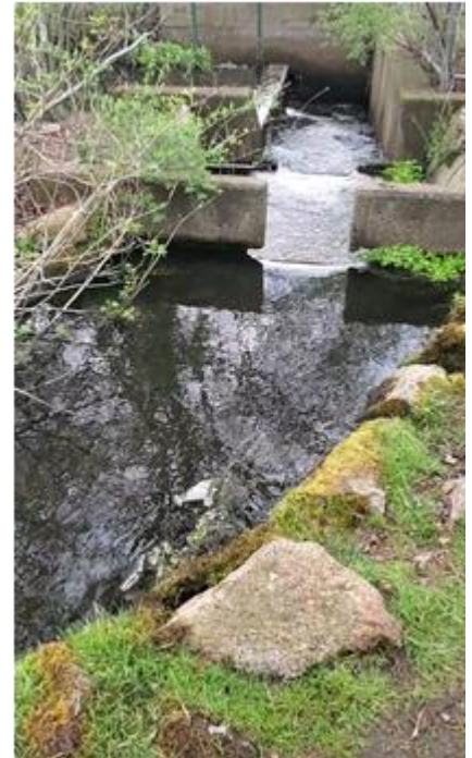
Worn steps and pools along fish ladder.
