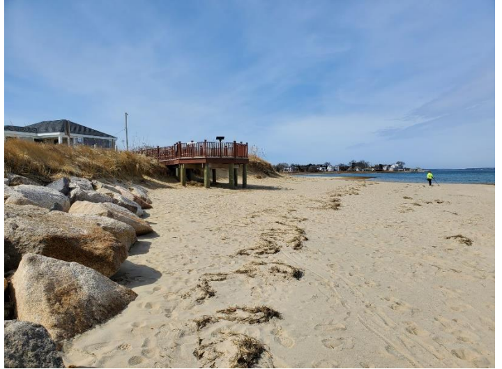
Storm Damage eroded sand underneath the observation deck after Winter Storm Keenan (Picture taken March 2022)
