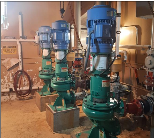
Photo 3: Bearse's Way Pump Station
