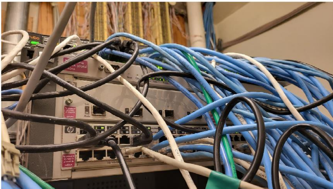
Example of Outdated Network Switch in Town Hall
