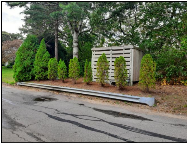
Photo 2: Estey Ave Pump Station
