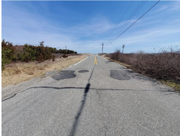
Asphalt and rock patches on Hawes Avenue due to broken culvert pipe under roadway (taken 3-15-2022).
