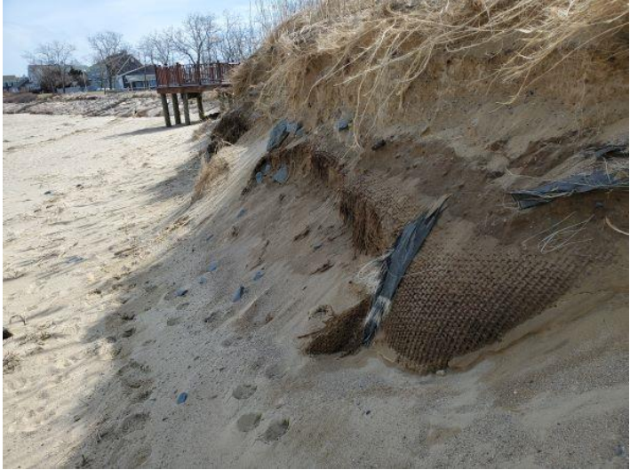
Storm Damage to Coir Roll System after Winter Storm Keenan (Picture taken March 2022)
