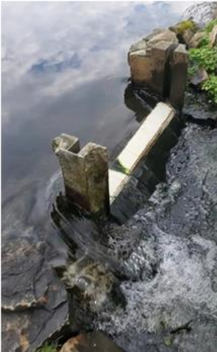
Stone damage and missing stones around the water control structure. Taken on 4/28/2021
