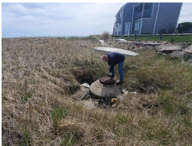
Junction manhole at the connection of an older culvert to a newer culvert that allows salt water connection to the upgradient salt marsh (taken 3-15-22).
