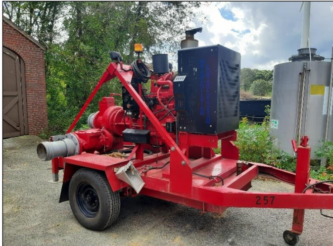
Photo 1: WPCD Bypass pump
