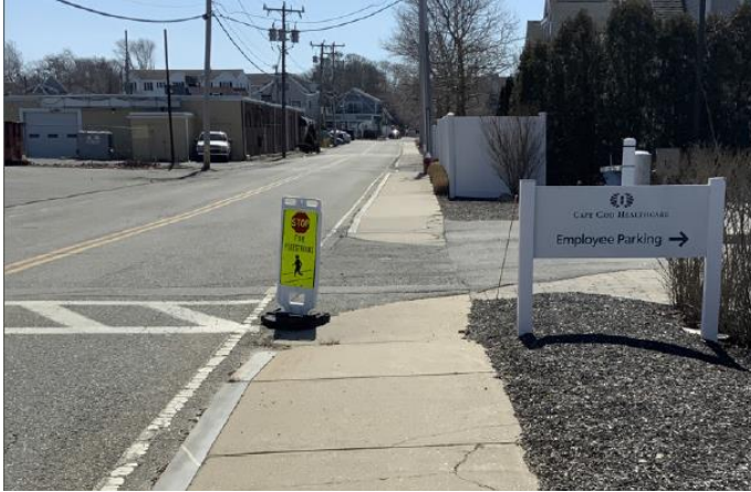
Exceeds allowable cross-slope pitch
